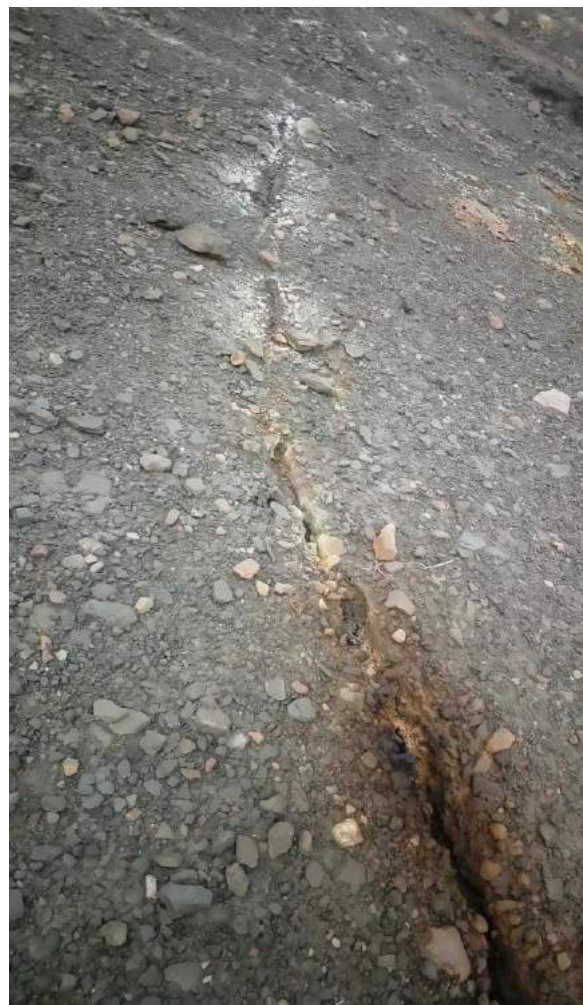
Figure 20: Fume cracks in the Bhulanbarari area.
